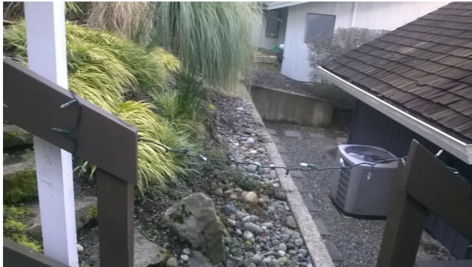
Figure 3. Area of proposed new watercourse buffer impacts. The proposed addition would extend 3 feet beyond the existing concrete retaining wall.
